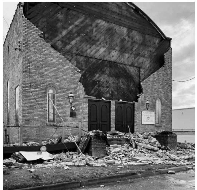
Hurricane Beryl damage to Congregation K’Nesseth Israel.
